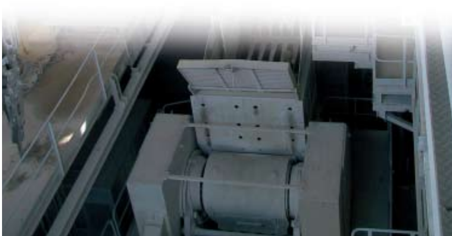
A C200 after replacement of a double toggle jaw crusher. Plant capacity was increased without having to modify the foundations.
